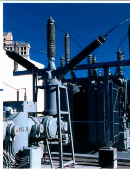
One possibility to connect GIS and transformer: outdoor-immersed bushing
