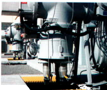
Field-proven cable connection to Nevada Power's network
