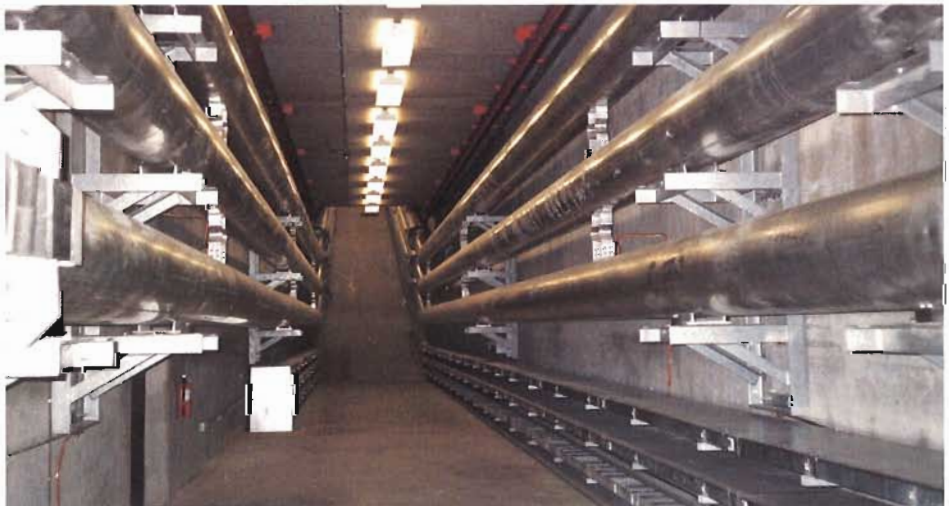
500kV, 4000A CGIT in a tunnel (Revelstoke B.C. Hydro, Canada)
