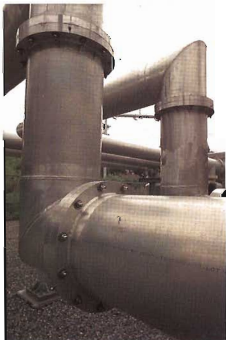
ABB's CGIT is designed to accommodate sharp changes in directions.
