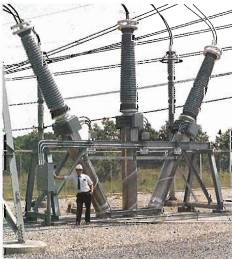
362kV, 4000A SF 6 Busduct with SF 6 -to-air bushing (Dunwoodie Substation, Consolidated Edison of New York)
