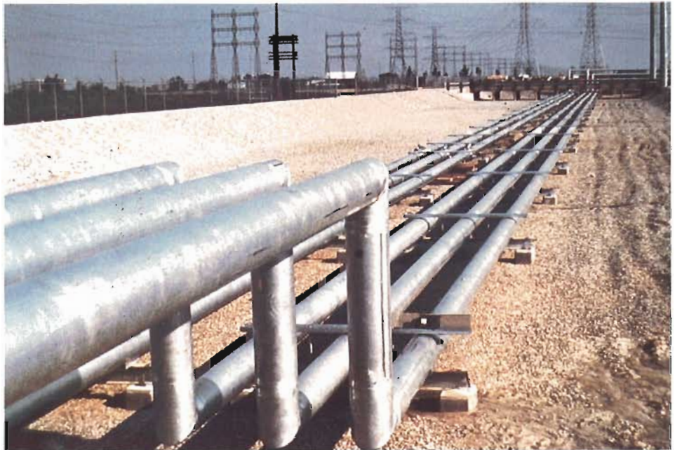
242kV, 3000A, Substation (Claireville, Ontario Hydro, Canada)
