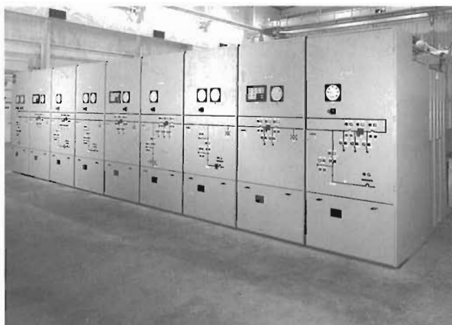
Picture 3 The line up of the 69 kV SF 6 -insulated cubicles shows on the front of the cubicles the single line diagram with local control components.
